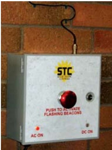
Figure 2, typical wall mount radio transmitter unit with roof-mounted antenna
