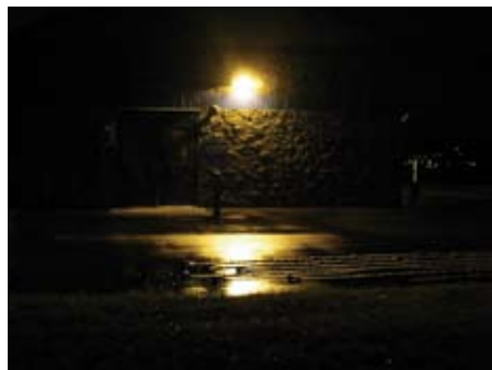
200 Watt, HPS wall pack. This luminaire produces a high amount of glare
